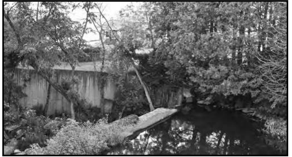
The blocks of the dam, eroded by years of moving water, have slowly lowered to allow more and more water through.
