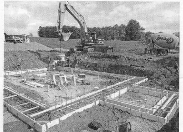
The footing was poured, including the addition for the bell tower which will be on the road gable end, and contains stairs from the basement to the second floor, which will meet fire and safety codes for a second exit. We know the bell tower was there from journal entries by former students. It was open, because ringing the bell for funerals was a cold job. And also, some students brought a sheep up to the top, and then lowered it out on a rope.
