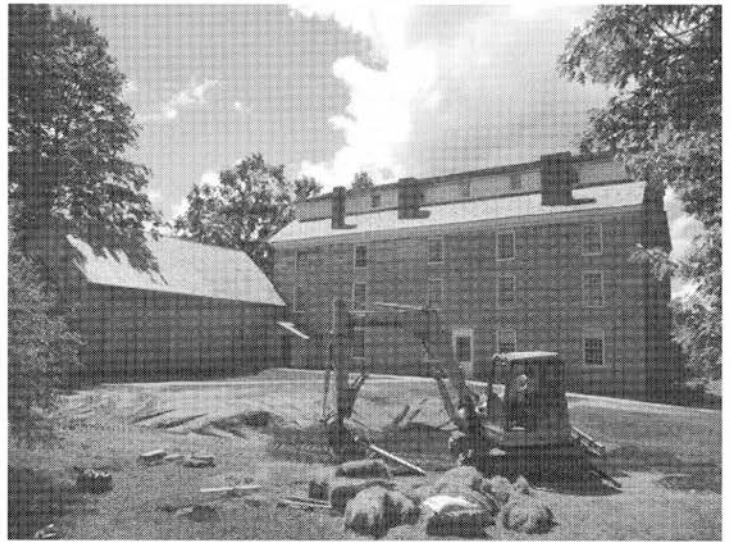
John and Johnny Rodgers built and packed earthen ramps to replace the wooden handicapped ramps leading into the Old Stone House and the adjoining barn. They seeded and mulched the new ground, and the summer rain has turned it into a nice lawn.
