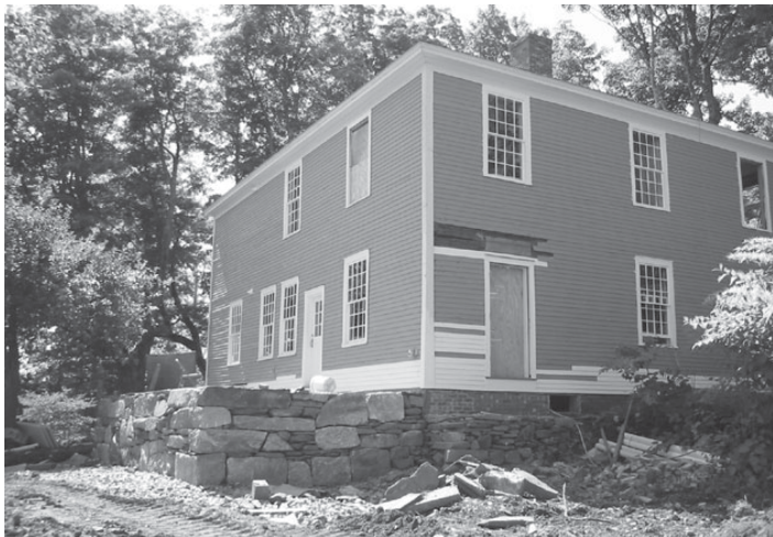
The northeast view of the Hall House shows the new stone terrace built by John Rodgers.
