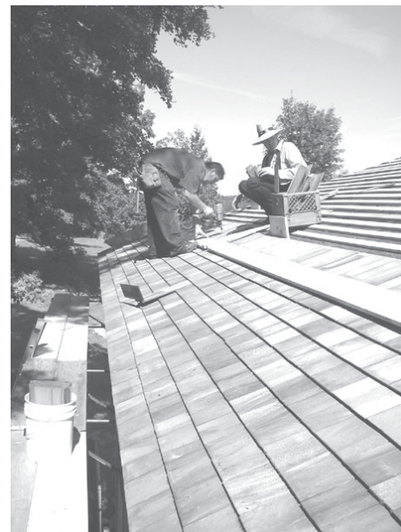
Ben Barnes, left, and Jim Daniels, right, have a stretch of sunny weather to put the fire resistant cedar shingles on the roof.
